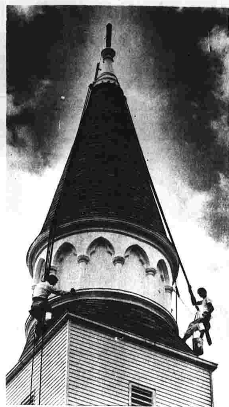
Steeple gets painted John Gresh, left, and Benjamin Charles of the Michael J. Gresh Painting Co. of Unionville are supported by ropes while painting the steeple of St. Bridget Church. The cross, missing in this photograph, is now atop the steeple, which is in the process of being refurbished. (Herald photo by Dunn)
